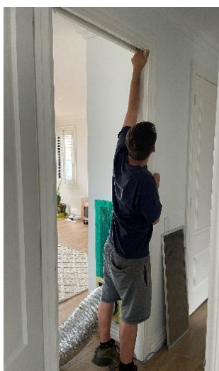
During testing, air could be felt from areas not considered "ductwork"
