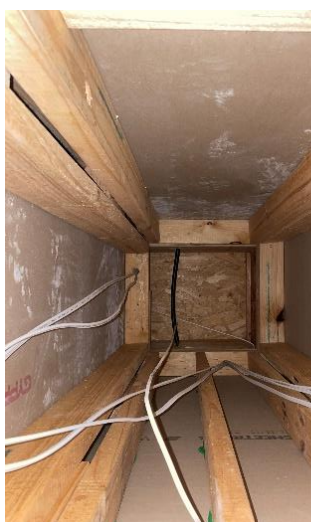
Building cavity leading to second floor
