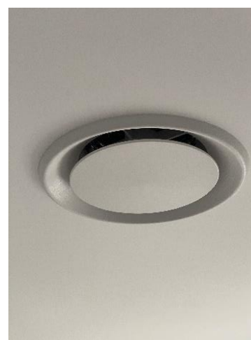
Ceiling vent with remote in-line fan
