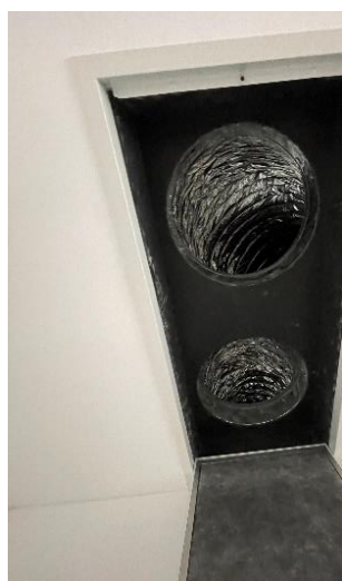
Systems with a ducted return generally performed better
