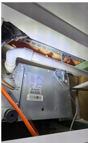
Insulation visible above unit, showing poor isolation
