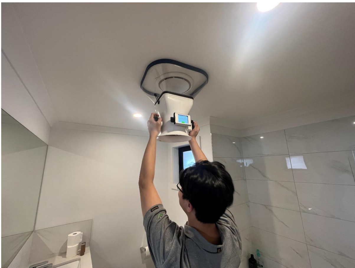
Figure 31 Measuring exhaust fan ventilation
