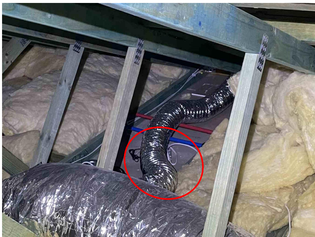
Figure 34 Crimped excess exhaust fan ductwork
